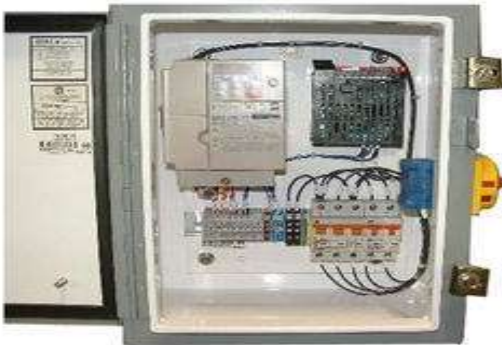
Fig.4 VFD Control Panel
